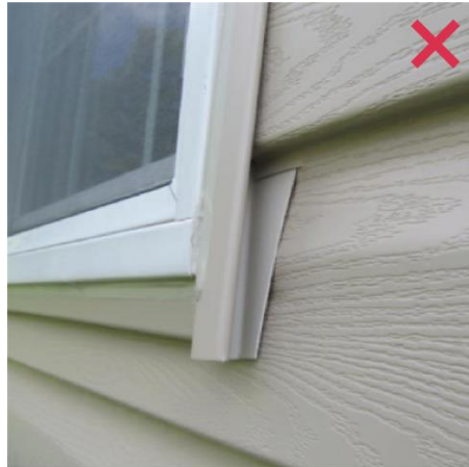
Figure 3: J-channel siding trim at the edge of an off-shelf clapboard cladding system prohibited. Proper trim required.
